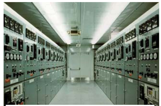
Power Distribution Center
